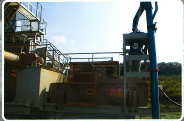
Cyclone & Fines Sand Screen
